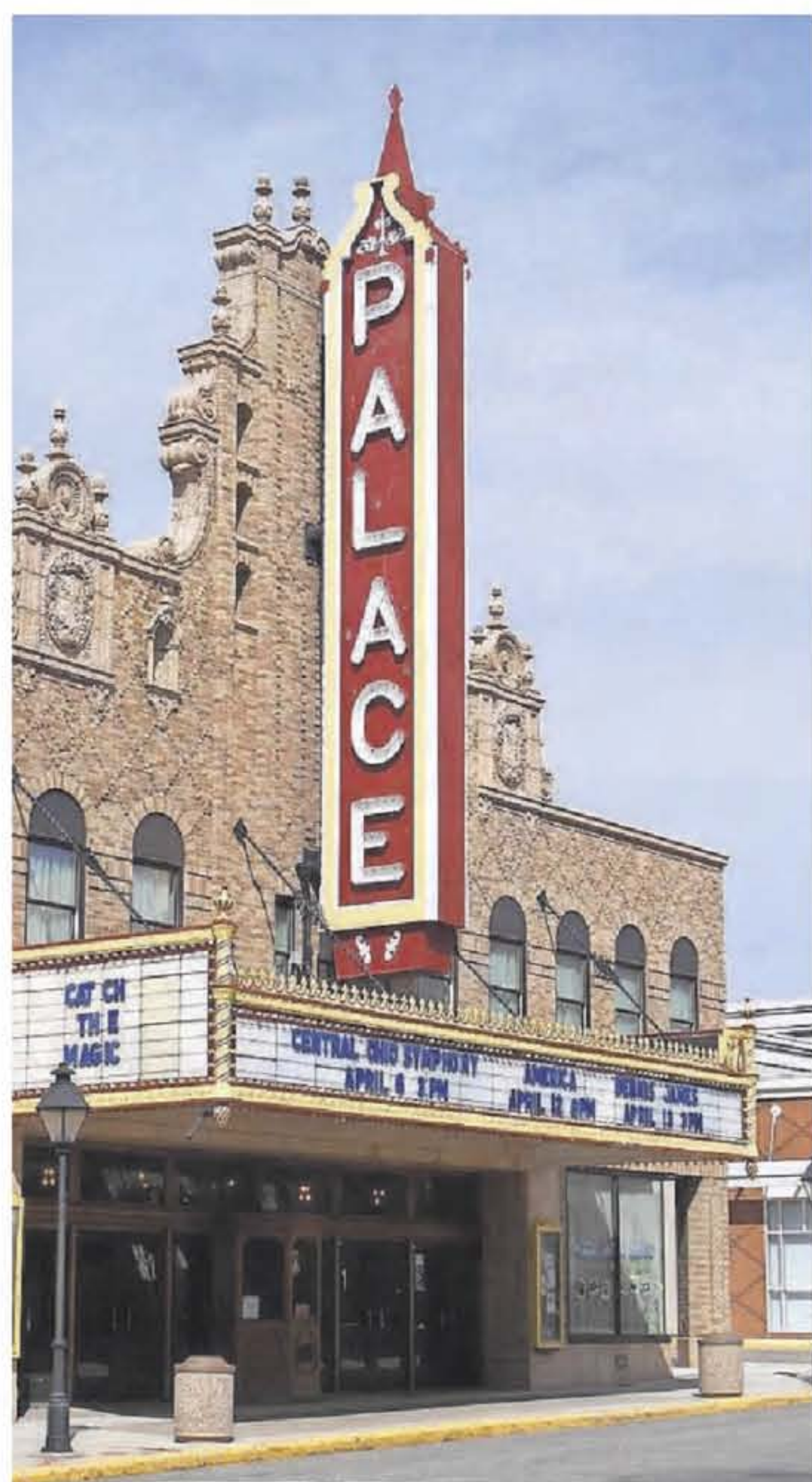
A local fund raising campaign helped fix the Palace Theatre’s deteriorating steel structure in 2013.
