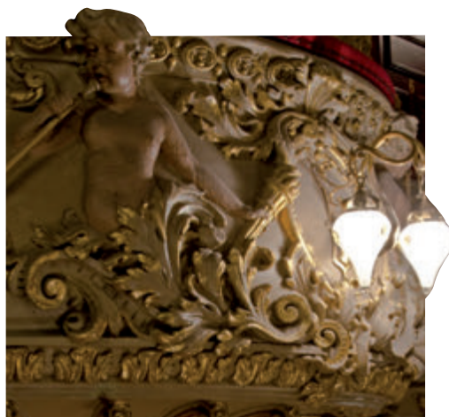
Pictured from left: main facade following restoration; new seats and carpet; restored foyer ceiling; restored ornate plasterwork on boxes. Images © M. Wolchover
