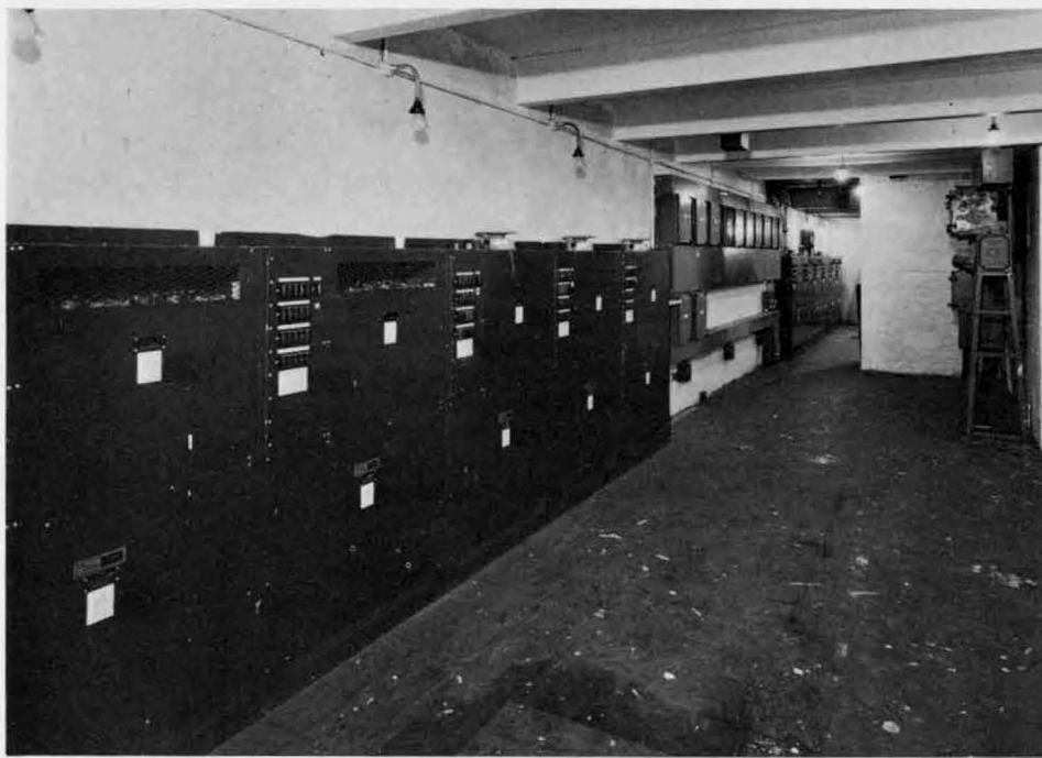
Dimmer room showing STM racks and the vast space vacated by the electro-mechanical banks.
